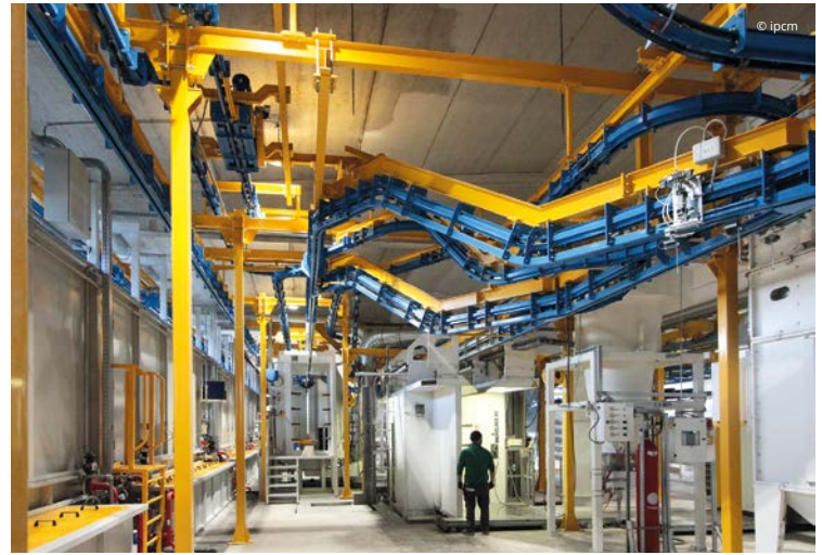
The application area, with a focus on the switches of the power&free conveyor supplied by Futura Convogliatori Aerei (Robecco Pavese, Pavia, Italy), which create the storage buffers needed to guarantee the flexibility of the system.
