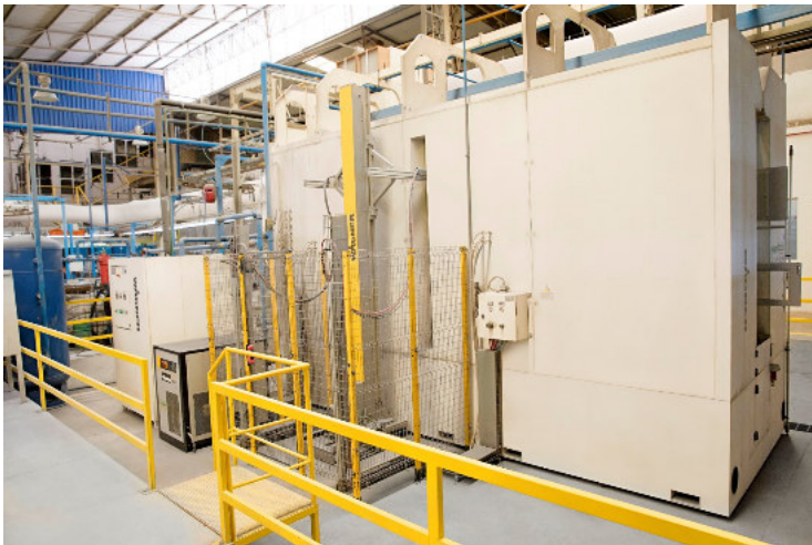
Backside of the powder booth with reciprocator and air treatment system
