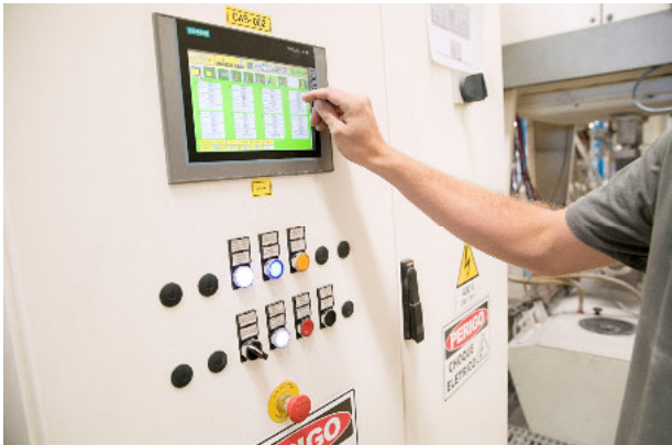
Central panel for the management of the complete booth system, including the automatic guns
