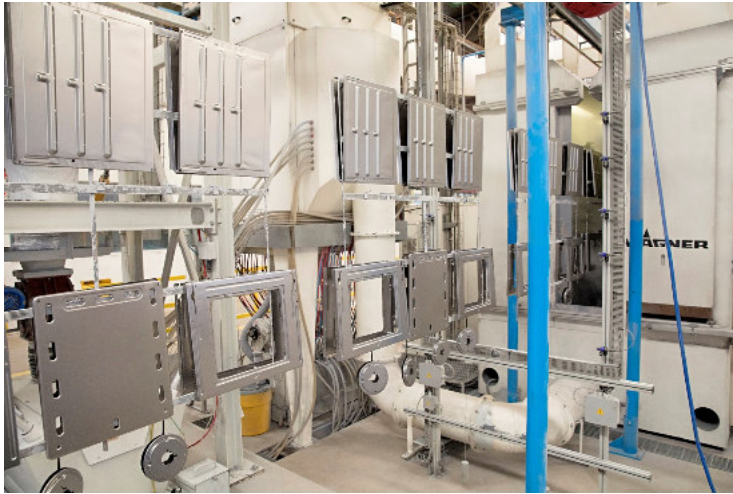
Workpieces at the entrance to the WAGNER enamel coating booth. A sensor captures the exact dimensions of the workpieces to determine the exact positioning of the automatic guns, thus enabling highest application efficiency and more economic use of enamel powder.
